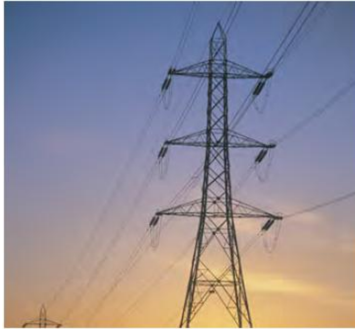
Figure 46 - Power lines carry a strong alternating current, which means that a substantial amount of charge is accelerating back and forth and generating electromagnetic waves. These waves can produce a buzzing sound from your car radio when you drive near the lines
