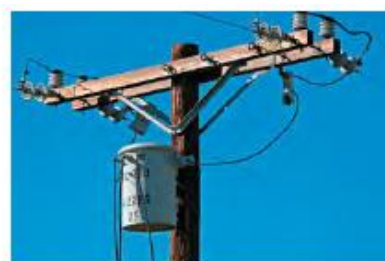
Figure 66 – The cylindrical can near the top of this power pole is a step-down transformer. It converts the high-voltage ac in the power lines to low-voltage (120 V) ac, which is then distributed to the surrounding homes and businesses
